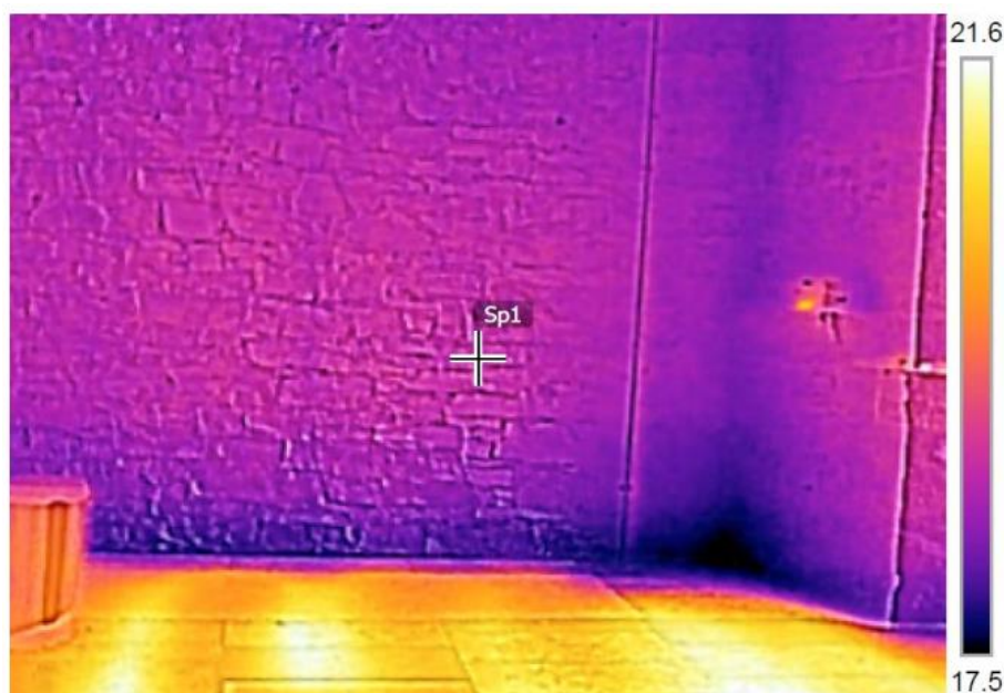
Figure 3: Thermal image showing additional heat flow at vertical and horizontal junctions with the abutting walls and floor. Note that the corner is the coldest point because it loses heat in three dimensions
