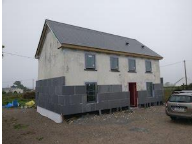
Figure 4: Examples of retrofitted traditional buildings, source: "Ballinahown, Co. Galway Deep Retrofit Case Study," Kore System. Available online: https://www.kore-system.com/case-studies/ballinahown-co-galway-deep-retrofit-case-study/ . [Accessed: June
