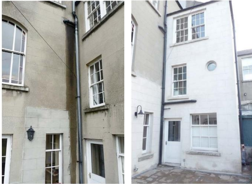
Figure 2: The same building with fixed drainpipe leak and cement render replaced with a traditional moisture-permeable lime render, source: "Energy Efficiency in Traditional Buildings"
