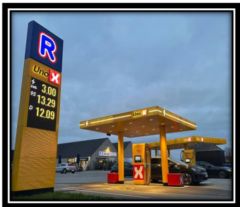
Fast EV Charger
