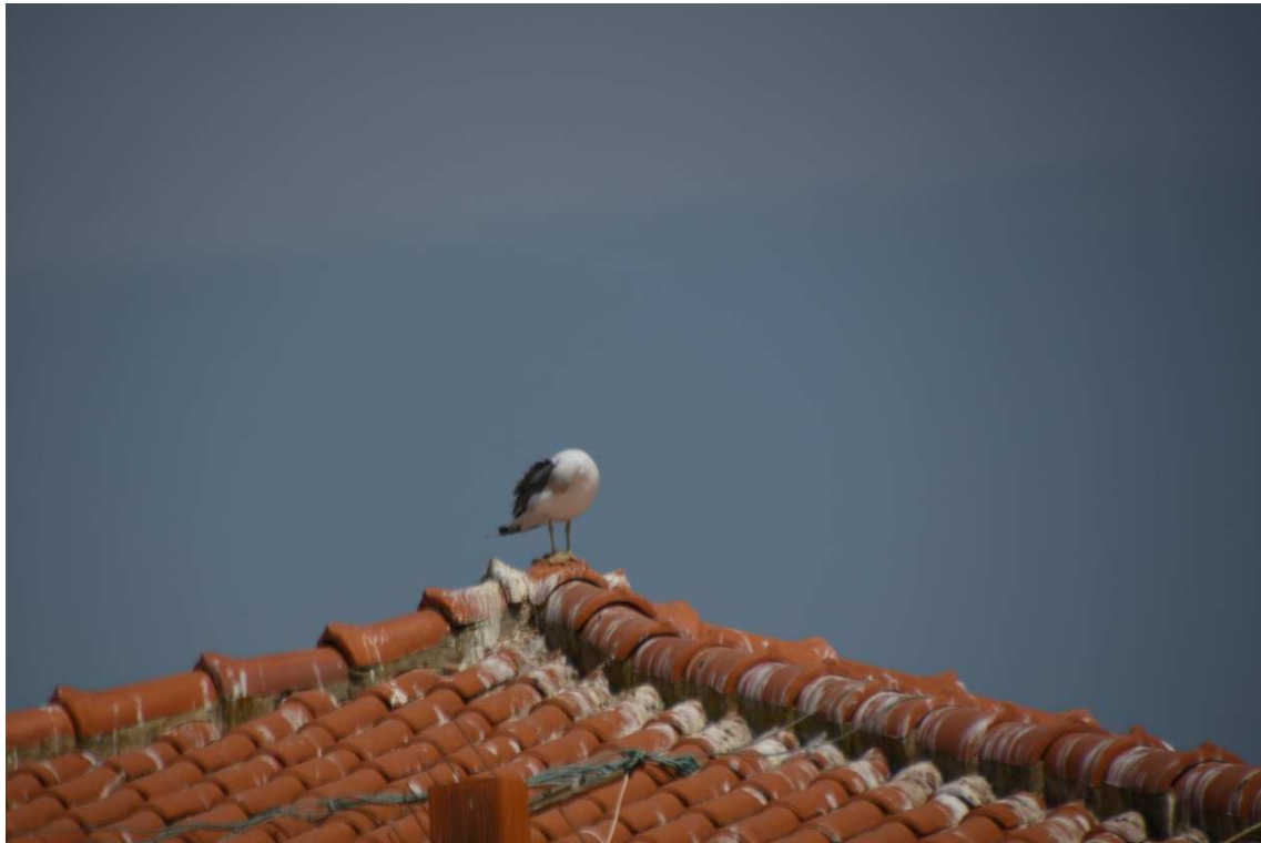
Figure 15: Soiling affecting the roofs - sports/community centre - bird droppings. please refer to Yield Calculations.
